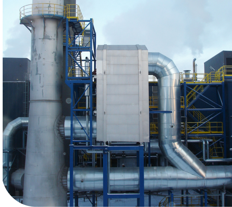
The second Aalborg AV-8N WHR boiler at the Tornio plant.
